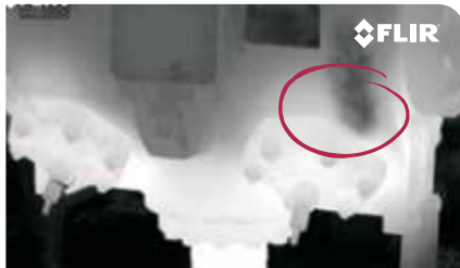
Captured gas leak.
