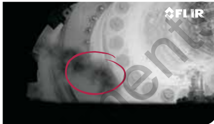
A leaking flange.
